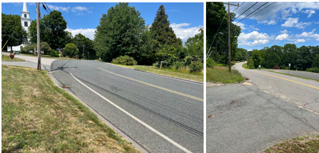
Existing shoulder lines on South Rd (left) and lack of shoulder lines on North Rd (right)
