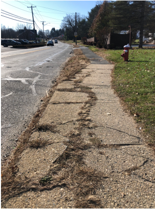
The sidewalks of SR-32 are cracked and impassible in places
