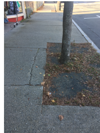
Exposed street tree pits may pose a tripping hazard to older adult pedestrians
