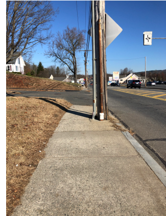
Utility poles narrow the width of the sidewalk, making it difficult to navigate for persons in wheelchairs
