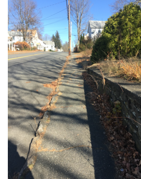
The Church Street sidewalks are narrow and cracked in places
