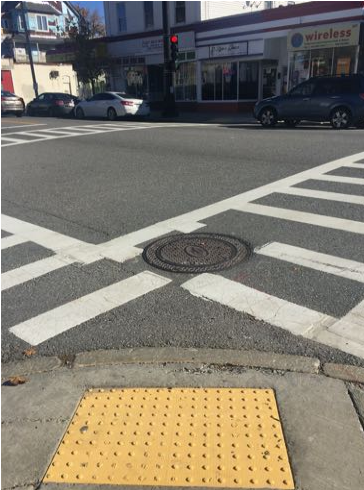
Misaligned tactile warning panel at Harlow Street intersection
