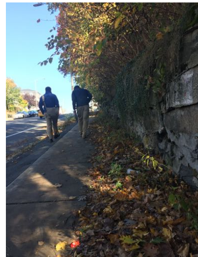
The east side sidewalk of Lincoln Street is sloped in sections and is obstructed by overgrown vegetation and fallen leaves
