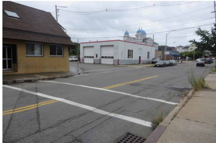
Crosswalks that lack ADA compliance and highly visible ladder designs are prevalent throughout Walnut Street.
