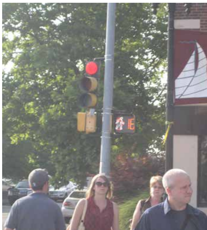
Malfunctioning pedestrian signal at Greenwood and Beale
