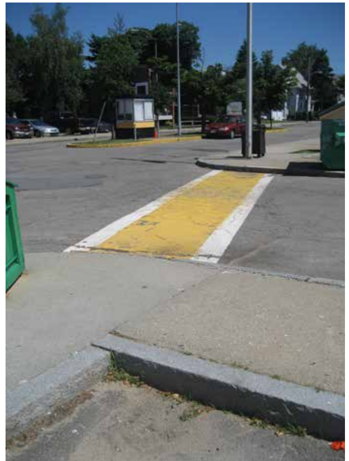
Sidewalks missing curb ramps at the parking lot entrance
