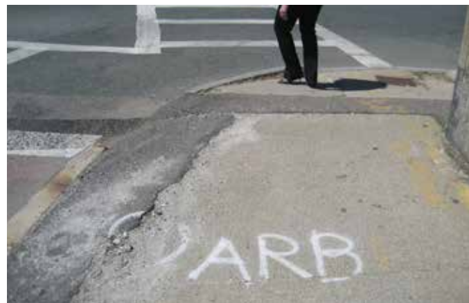
Patched sidewalk with no curb ramps at the corner of Newport and Beale
