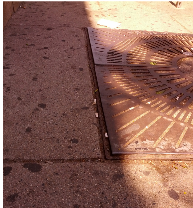
Popped tree grate
