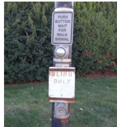
Figure 8: Separate pushbutton provided at Mount Auburn Street and Irving Street to activate the audible signals.
