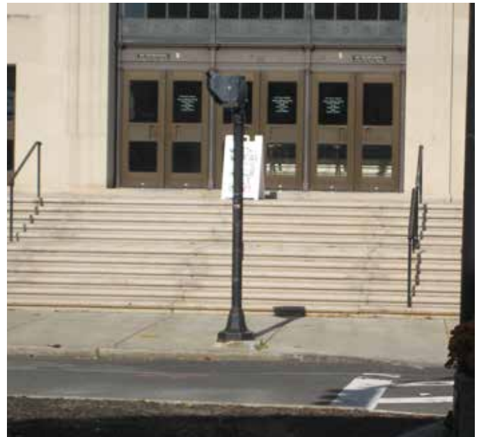
Misaligned pedestrian signal at City Hall Square
