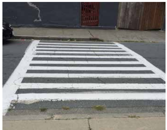
This high visibility crosswalk near the Gomes School has no curb ramps or detectable warning panels.
