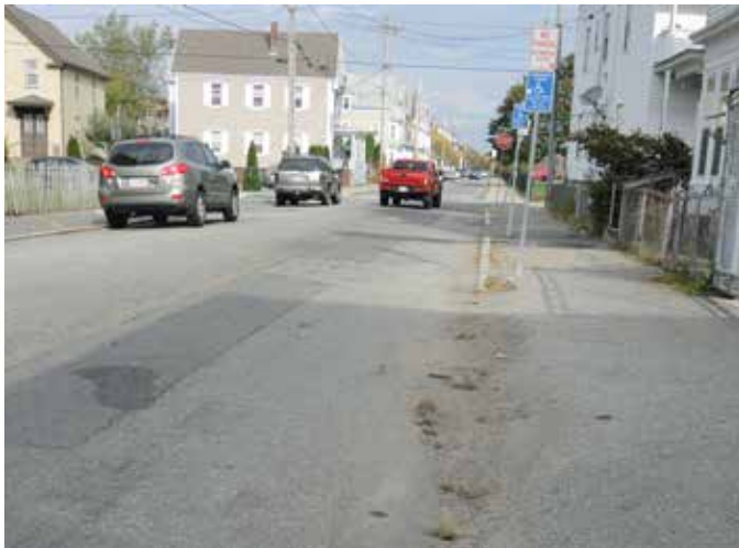
Asphalt sidewalk on along S 2nd Street between Rivet and Potomska Street
