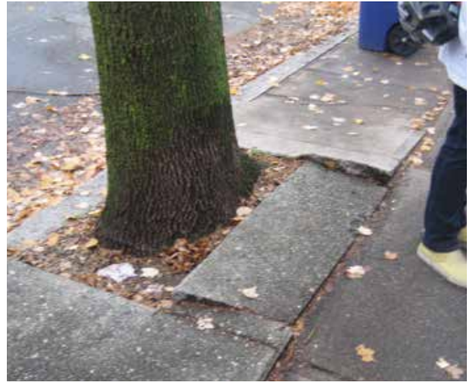
Heaving concrete panels around trees are tripping hazards.
