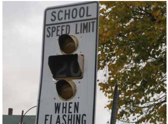
The school zone beacon at the intersection of Pearl and Cross Streets is not functioning
