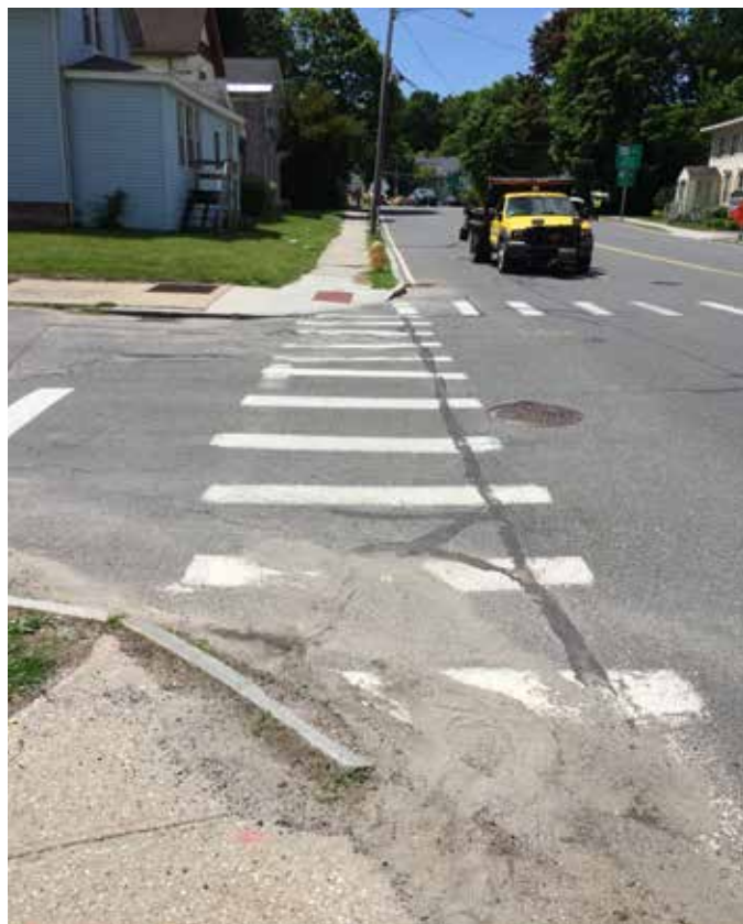
Broken curb ramps, sidewalks, and debris make this intersection an unwelcome crossing.
