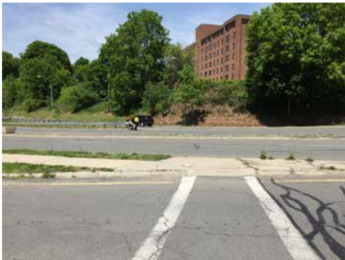
Cars coming from the access road onto Center Street do not yield at this crosswalk, which is poorly painted and not well signed.
