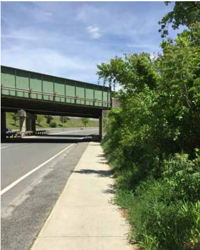
Example of a high-risk, unattractive road segment
