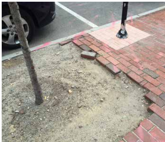
While the Main Street sidewalks are generally in good shape, there are ongoing maintenance issues with brick sidewalks that can create tripping hazards
