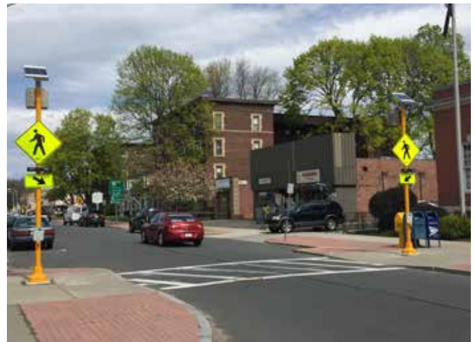
Rectangular Rapid Flash Beacon (RRFB) in West Springfield
