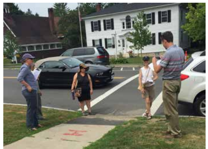
Crosswalks on Main Street need tactile warning strips and ADA-compliant curb ramps
