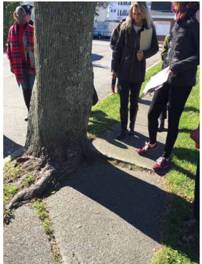
Trees have uprooted concrete sidewalk panels along all sides of Ashley Park. Sidewalks - in general - have not been upgraded in this area in several years.
