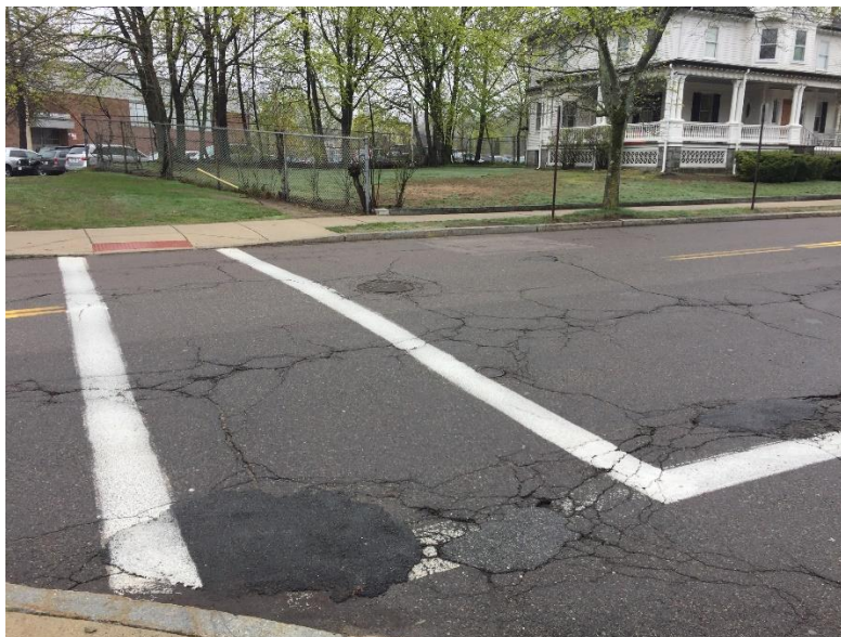
Crosswalk at Ashland Street does not meet current standards
