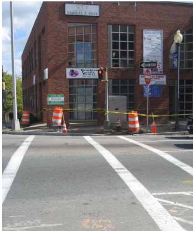
Lack of pedestrian accommodations during construction at the intersection of Main Street and Pleasant Street
